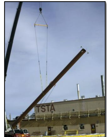
One of the unique aspects of the scope of work for this project was the demolition of a 60-ft. exhaust stack. EDi provided the site supervision, operators and laborers to execute this task. The stack was safely demolished and packaged for waste disposal.
