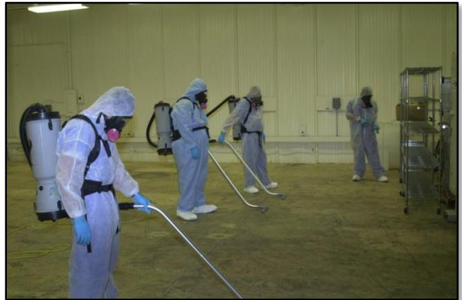
HEPA backpack-style canister vacuums used to decontaminate surfaces of beryllium project-wide.
