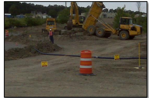
NRC-Licensed Disposal Area: Looking north at the Buffer Area ingress egress in foreground and soil mixing area in the center.
