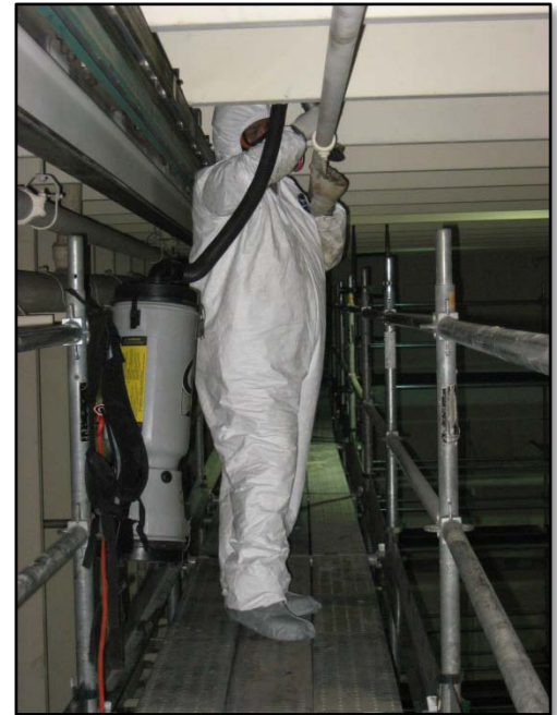
HEPA Backpack-style Canister Vacuums used to decontaminate designated buildings of beryllium dust at SNL/NM.
